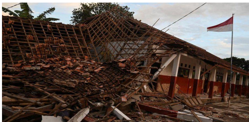
A collapsed school building in Cianjur
